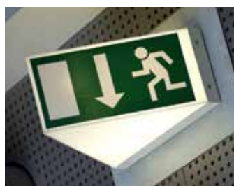
Safety lighting systems, emergency power supplies
