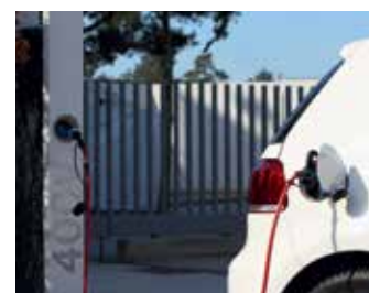
Charging stations for electric vehicles
